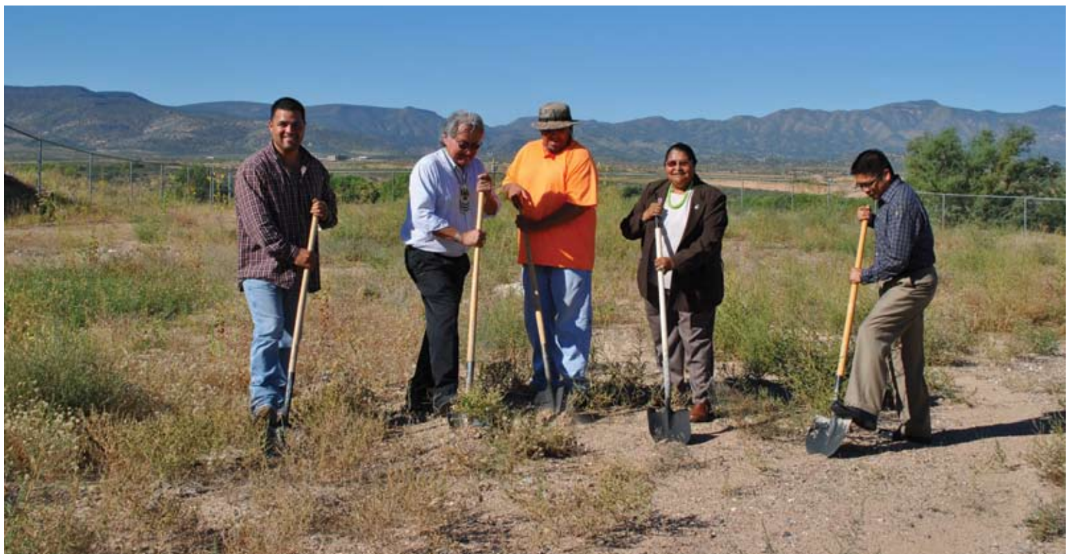
FROM LEFT TO RIGHT: YAC Residential Superintendent Matthew Bejarano, YAC Board Member Don Decker, YAC Equipment Operator Chad Bates, Councilwoman Linda Evans, YANTH Executive Director Rick Preston officially break ground on Sine Street.
